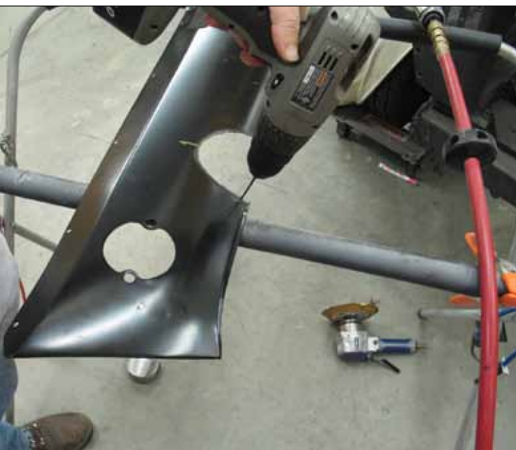
We used the surround studs and a paint marker to mark the holes for the surround. We used a small drill bit to form a guide hole then a larger bit to drill the final hole on either side of the surround.
